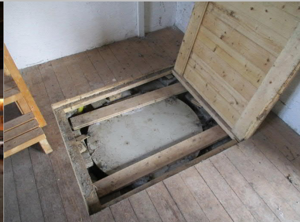
Synlig pumpgrop under plankgolv, bottenplan
