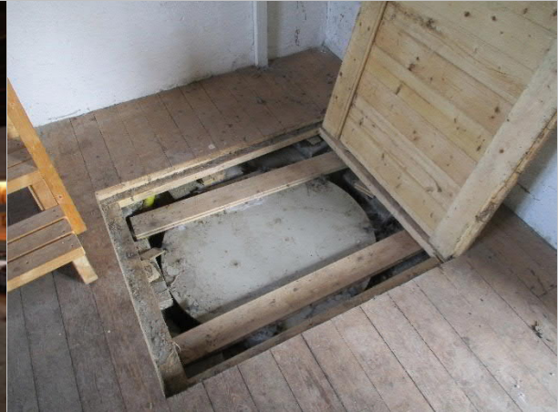
Synlig pumpgrop under plankgolv, bottenplan
